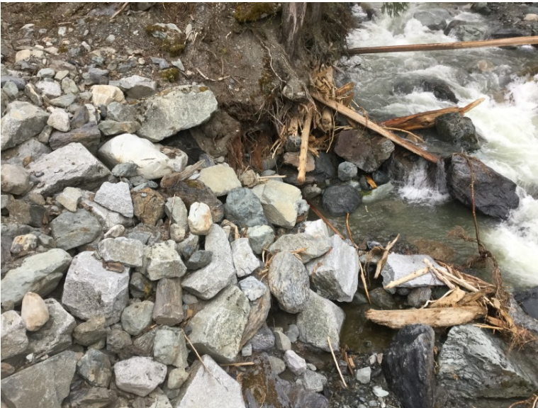
Upstream right bank riprap scour
